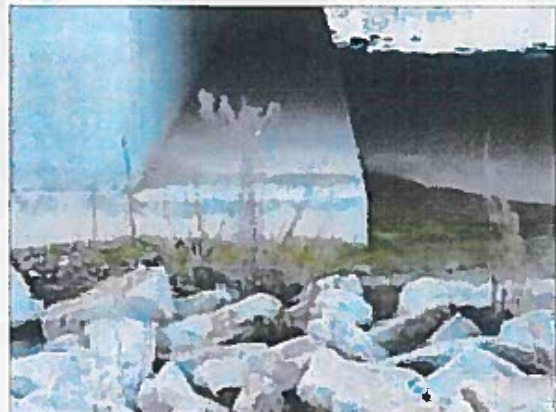
Pied-sec non conforme car vertical
